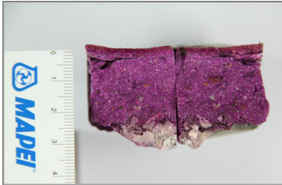
FIG. 20.8 - SAMPLE TAKEN FROM THE STRUCTURE AND ANALYSED WITH PHENOLPHTHALEIN: THE TOTAL ABSENCE OF CARBONATION IN THE CONCRETE THICKNESS CAN BE SEEN
